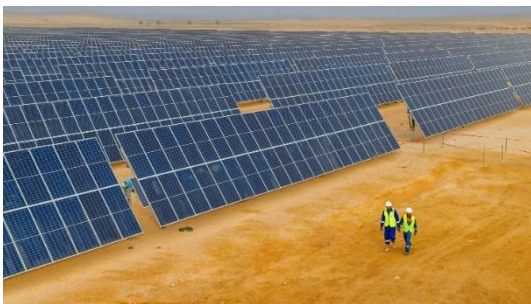
Figure 2. ENI photovoltaic plant in Tataouine.
